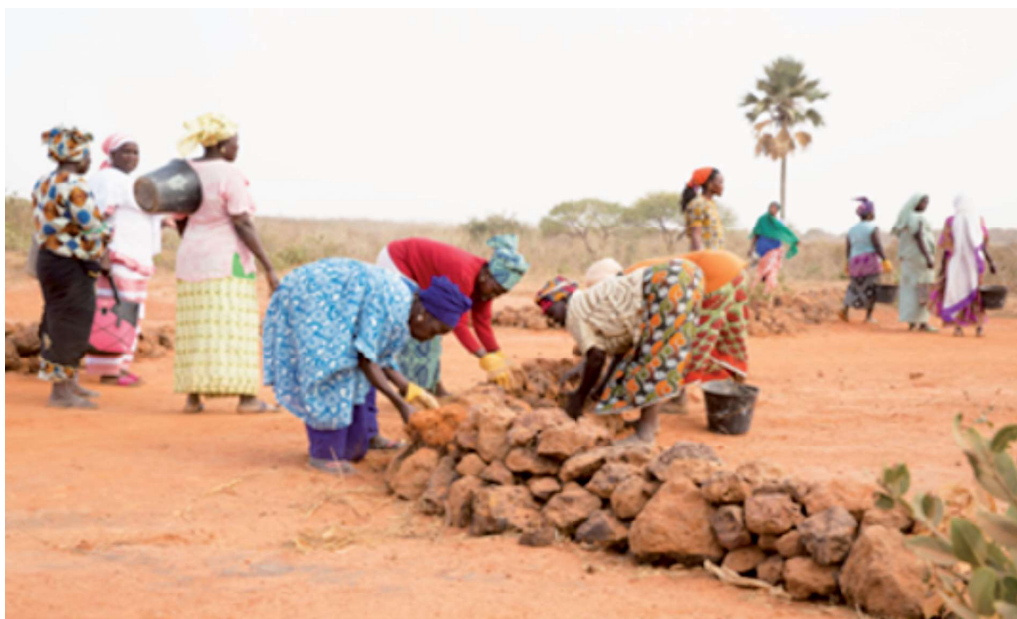
Development of a half-moon ground to promote water infiltration and the conservation of humidity in the soil around the trees
