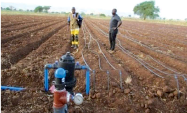
Solar powered irrigation system
